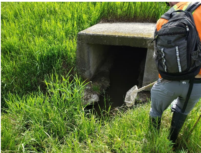
Photograph 31. ↑ C10-A-6, June 2022. Looking downstream (east) at Hwy 400 Culvert inlet. The concrete bottom of the culvert appears to have been eroded away.
