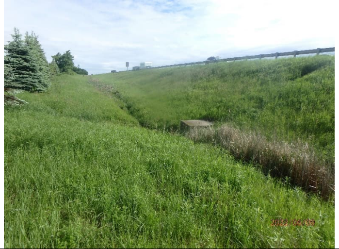
Photograph 30. ↑ C10-A-6, June 2022. Mapped feature within highway 400 RoW – looking at culvert inlet on west side of highway.
