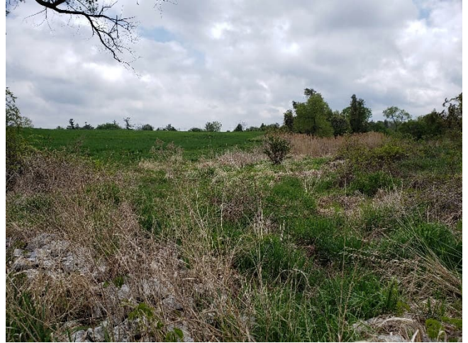
Photograph 178. ↑ C27-A-1, May 2022. Downstream reach bank with rip-rap and surrounding agricultural land use.
