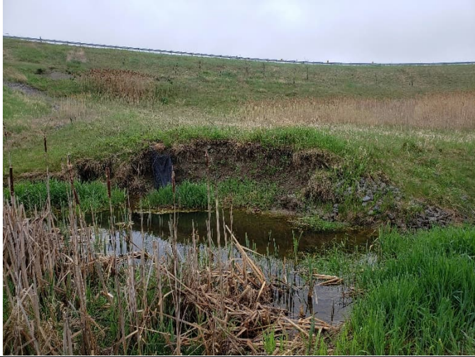
Photograph 181. ↑ C28-A-1, May 2022. Downstream reach facing left bank with active erosion.
