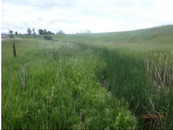
Photograph 29. ↑ C10-A-6, June 2022. Mapped feature within highway 400 RoW – looking downstream on east side of highway.
