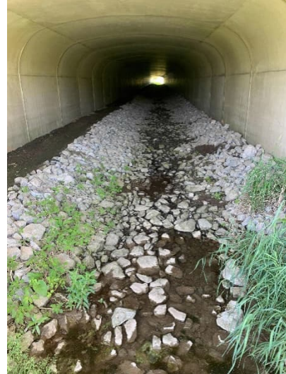
Photograph 174. ↑ C26-A-1, June 2021. Standing water in culvert on west side of Highway 404.
