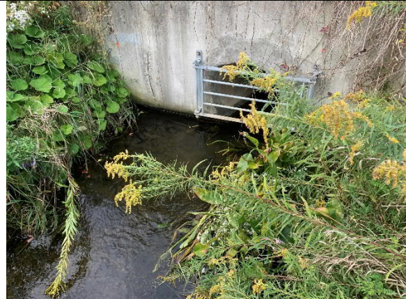
Photograph 6: SWMP outlet structure discharging into channel feature, west side of County Road 4.
