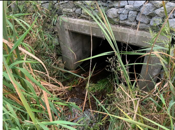
Photograph 7: County Road 4 culvert inlet on west side, dense vegetation growth around inlet.
