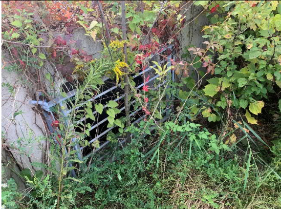
Photograph 5: SWMP outlet structure. Overgrown vegetation at overflow feature.
