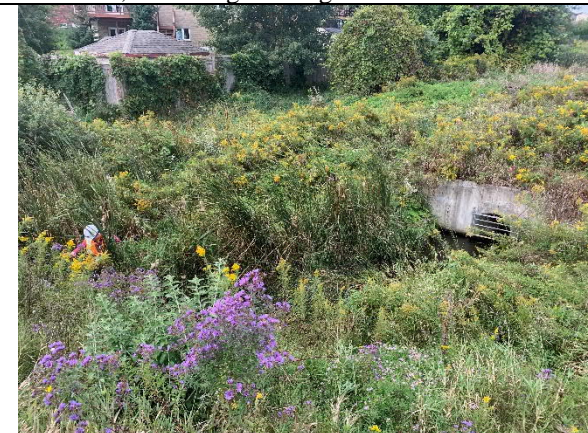
Photograph 9: Looking west from County Road for at channel section between culvert inlet and SWMP outlet.
